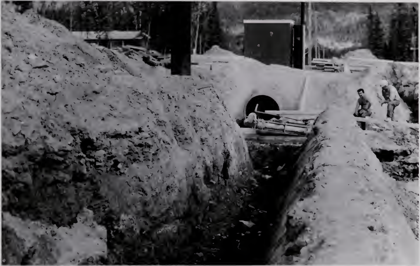
Plate 5. The utilidor at Clinton Creek. The photograph is taken toward the east and the valley of the Fortymile River can be seen in the distance. (July 1970).
